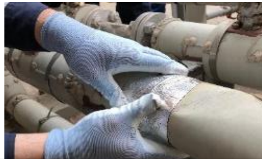
Firmly hand-pressing on uneven surface to put sufficient pressure on tape to ensure proper adherence.
